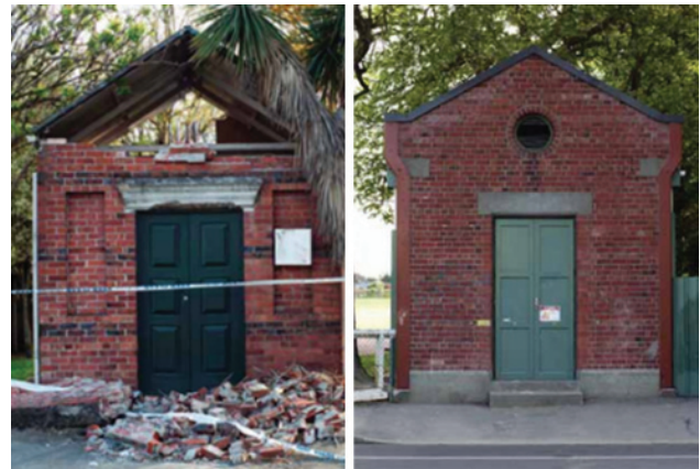
Figure 1 Substations belonging to the Christchurch’s electricity network [3]
