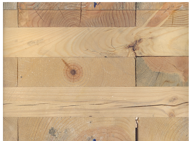
Figure 7 Checking, gap widening, material defect, and delamination in edge condition Specimen A, day 42
