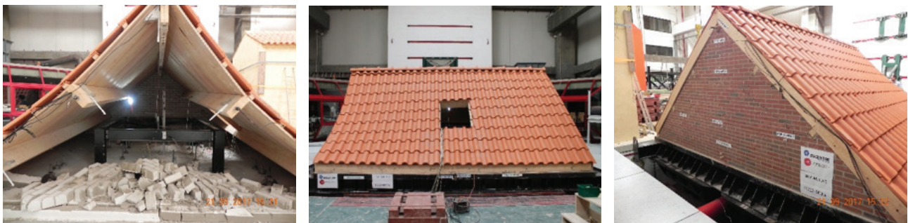
Figure 10 Damaged specimen at the end of test FEQ2-600%
