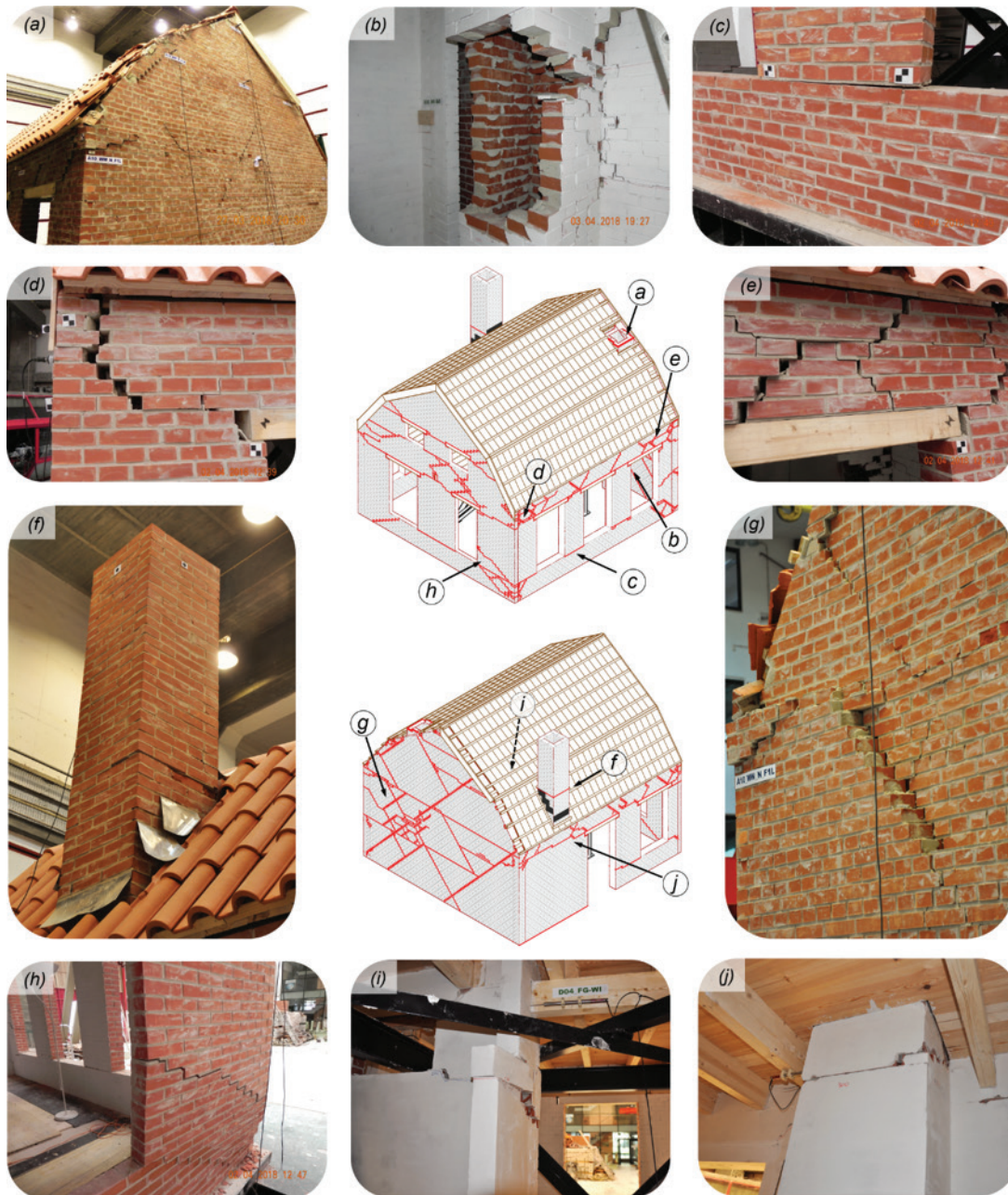
Figure 12 Observed damage after test SC2-500%: a) collapse of West façade chimney; b) collapse of the West chimney in the interior of the building; c) flexural crack at the base of a North pier; d) cracks at the top of the North wall due to out-of-plane mechanism of the East façade; e) large permanent openings on the North spandrels; f) cracking of the South chimney; g) mortar-joint sliding on the West façade; h) near-collapse state of the East façade; i) damage in the interior wall; j) horizontal crack at the base of the South chimney stack
